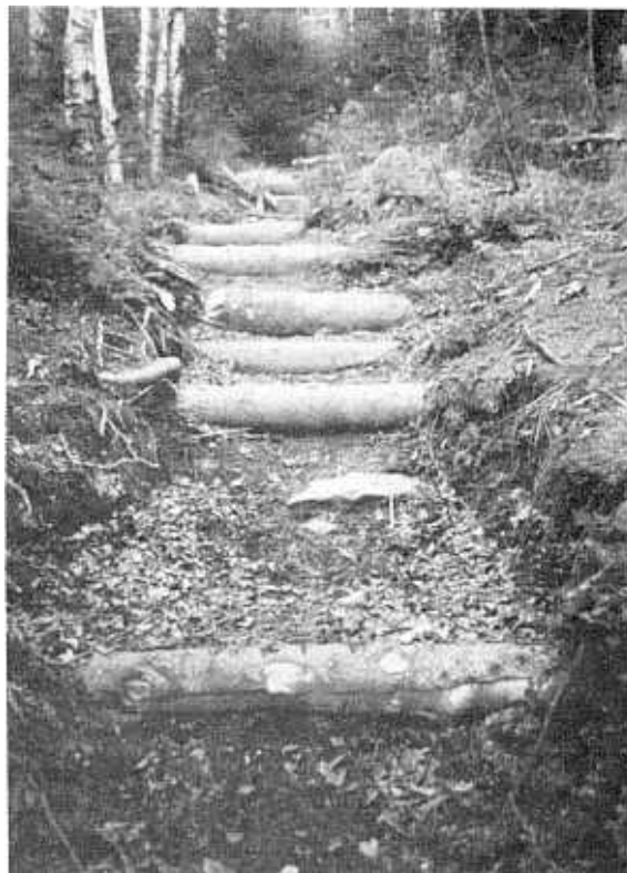
Initial repair work on the upper Walden Trail. Poor trail layout and inadequate drainage have resulted in serious erosion.
